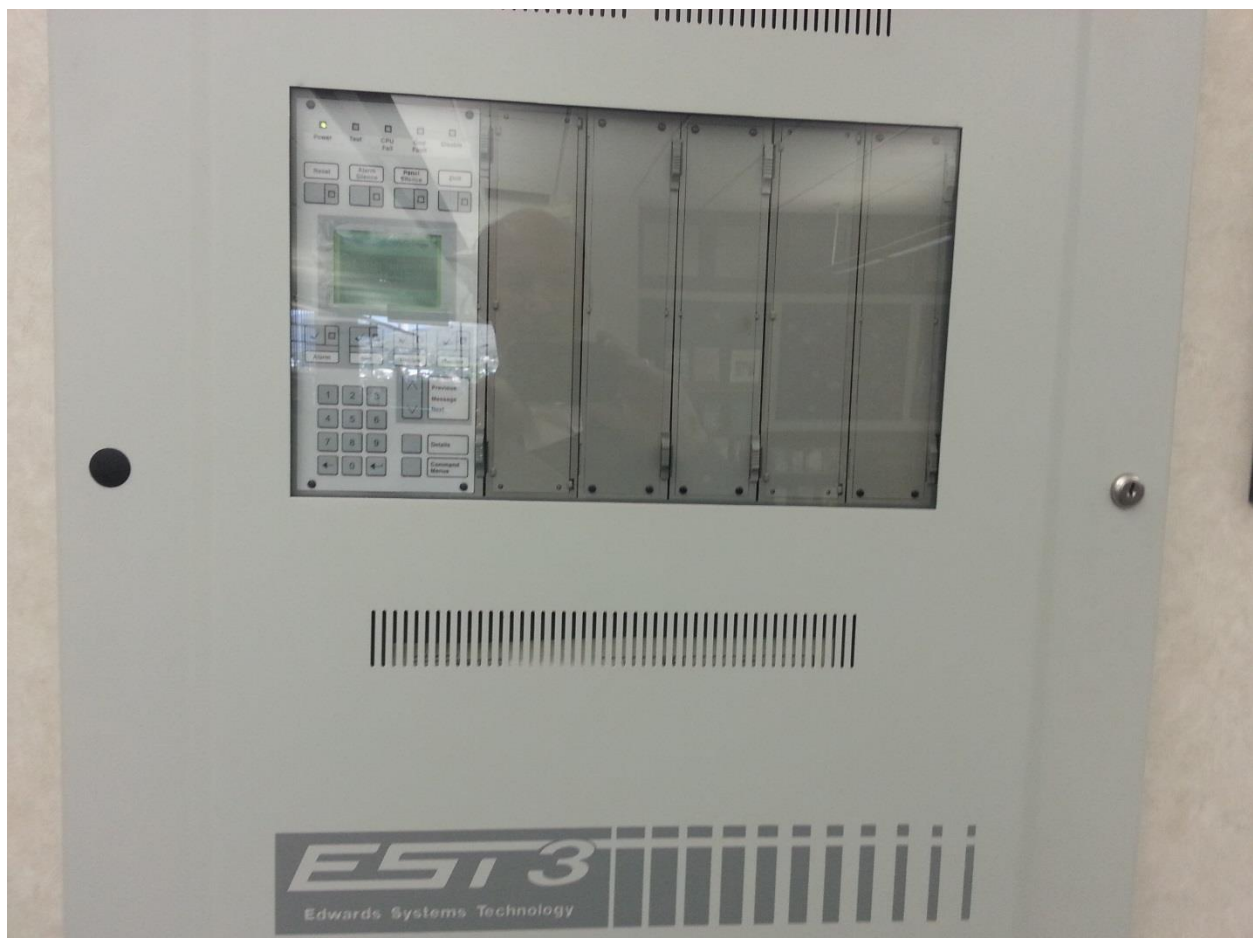
Existing Fire Alarm System
